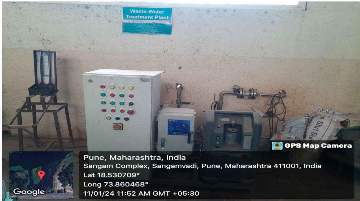
Waste Water Treatment plant installed in the Campus
