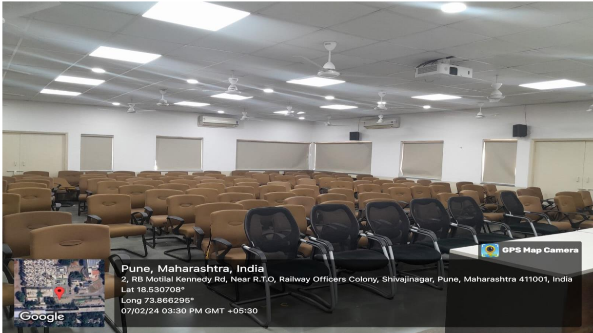
LED Tubes fitted in Computer Centre
