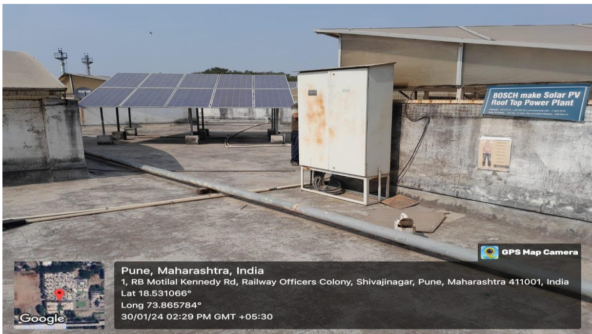
Solar Panels at Rooftop
