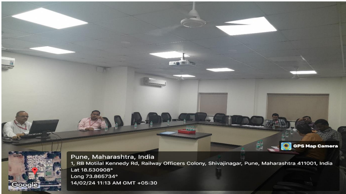
LED tube lights at the Conference Hall
