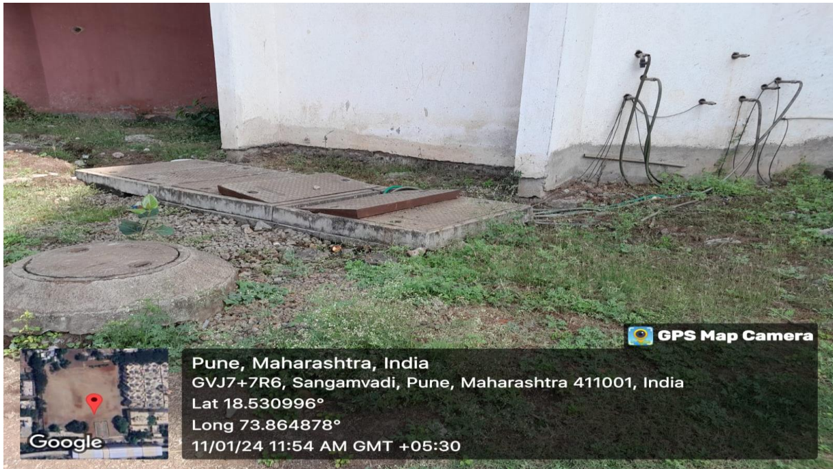
Tanks for the Water Treatment Plant
