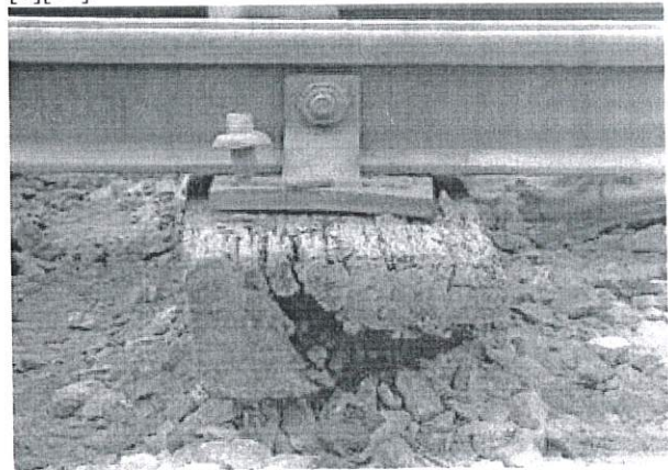
Fig. 1:- Fungal Decay of Timber Sleepers.
